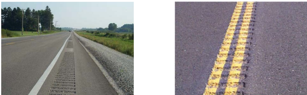
Figure A23. Example of centerline rumble strips (left panel) and shoulder rumble strips (right panel).
