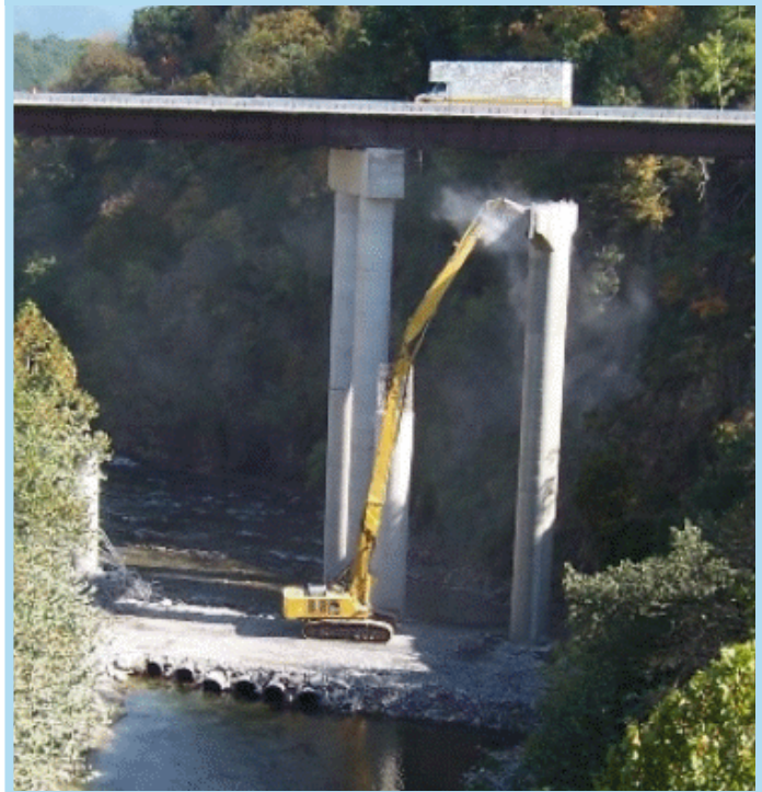
FIGURE 13 - ULTRA HIGH REACH EXCAVATOR ON DEMO OF SUBSTRUCTURE AT JIM THORPE BRIDGE
