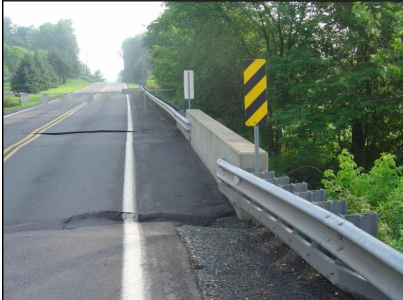
Settlement damage in the approach fill behind the abutments as viewed from the roadway above the bridge.
