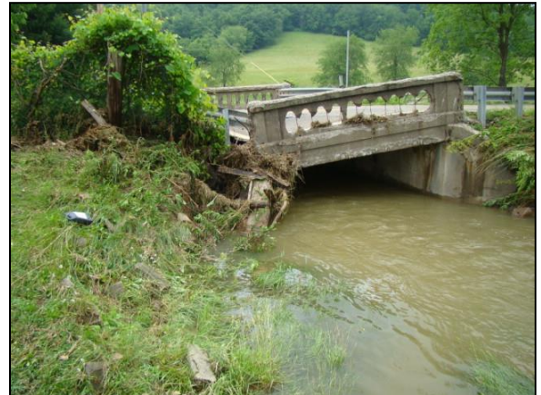
Settlement damage of the bridge causing tilt and roadway settlement damage in the picture to the left
