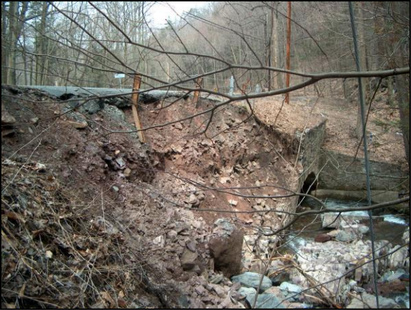
Embankment erosion damage and part of bridge has collapsed into the stream channel
