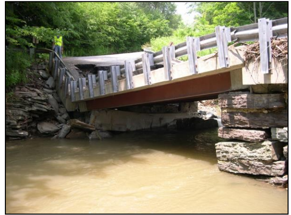
Extreme settlement damage in the abutment
