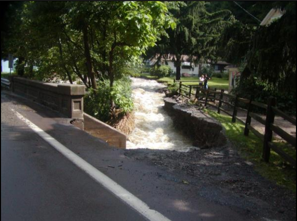
Embankment erosion damage under the adjacent roadway. The roadway shoulder has fallen away
