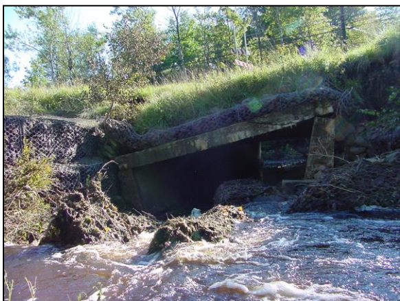
Settlement damage in the abutment due to scour underneath the bridge abutment
