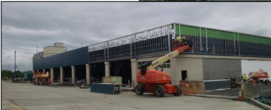
From top to bottom: New administration building, new parking structure, and bus storage facility
